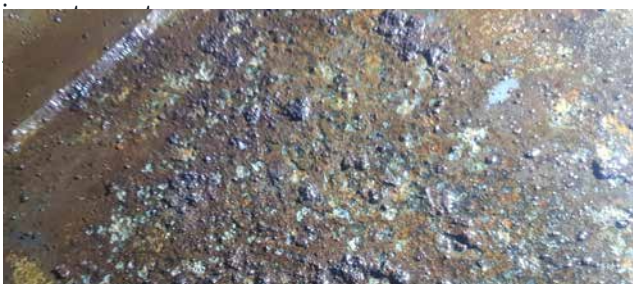
Corroded tank surface before Wolf tank Adisa operation
